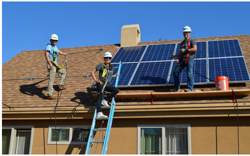
GRID Alternatives staff and volunteers install solar on one of the Triangle Court units.
