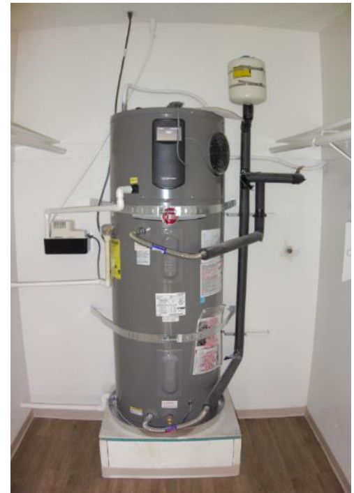
New in-unit heat pump water heaters replaced the existing aging electric resistance water heaters. Smart heat pump technology paired with renewable energy provides residents with increased energy bill savings.
