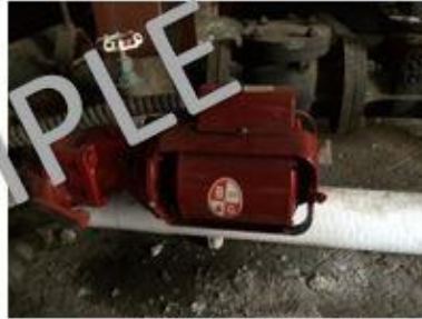
New Recirculation Pump
