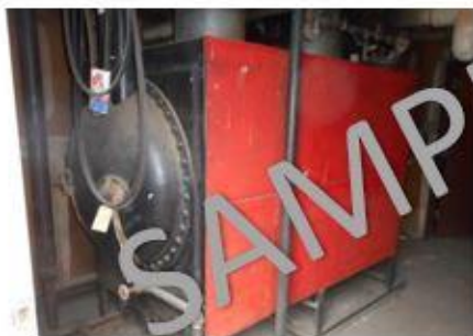
Existing DHW Boiler
