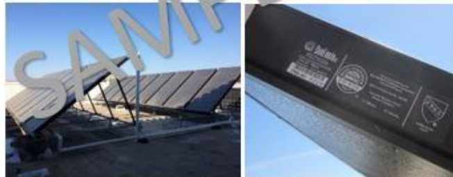
New Solar Thermal System
