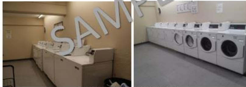
Existing and New Laundry Washers
