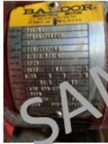
Existing Recirculation Pump
