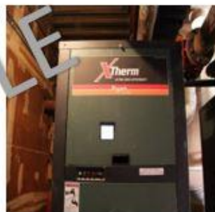
New DHW Boiler
