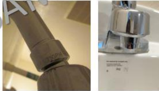
New 1.75 GPM Showerhead and 1.5 GPM Aerator
